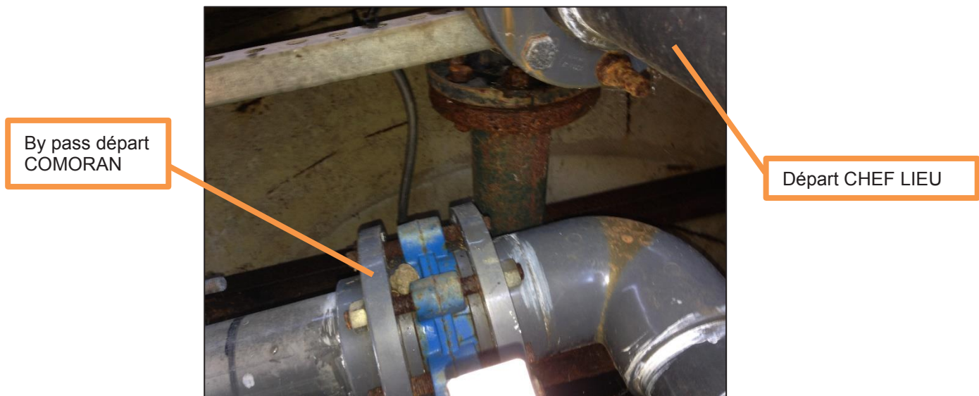
Figure 14 :Puits Agostini – Equipements
