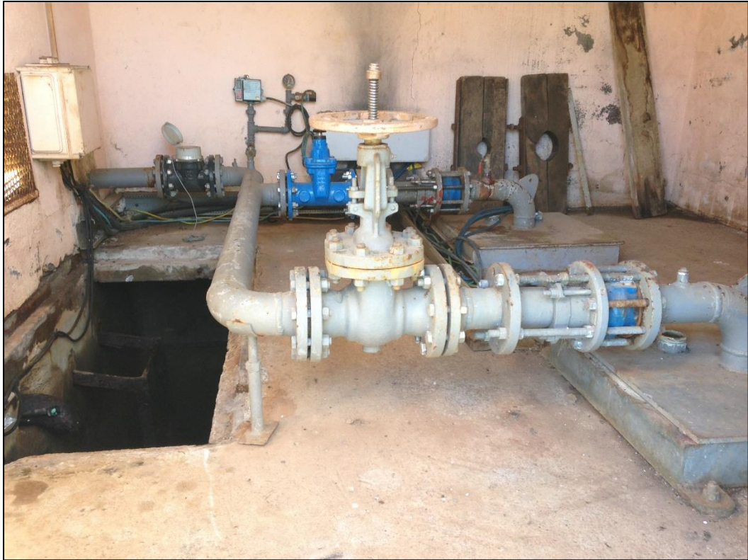
Figure 32 : Equipements station pompage
