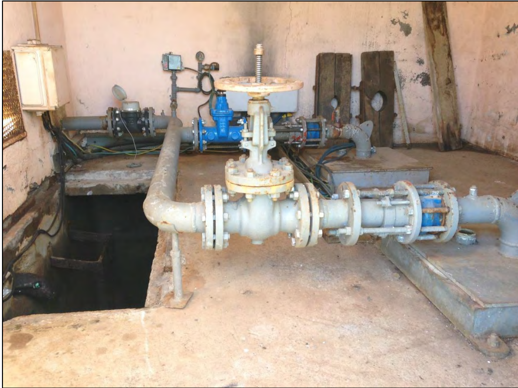
Figure 32 : Equipements station pompage
