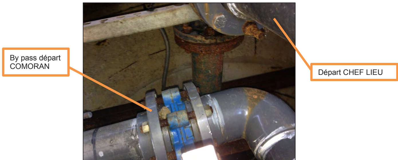
Figure 14 :Puits Agostini – Equipements
